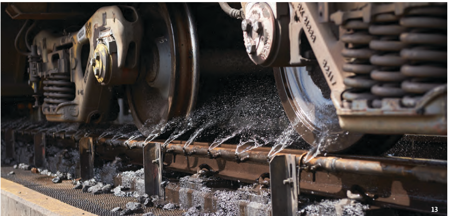
Wagon wheel wash infrastructure that minimises dust carried away by rolling stock following inloading.
